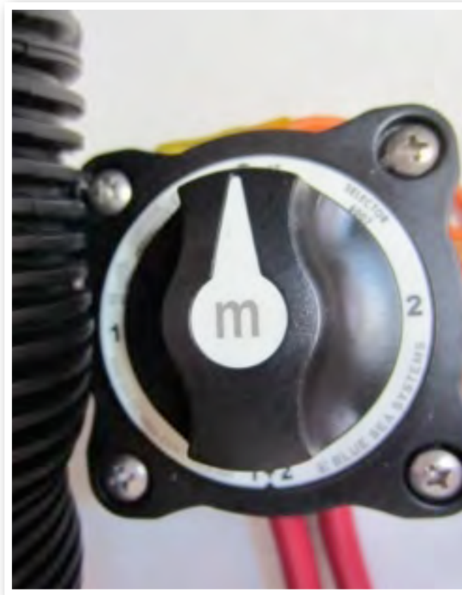
Battery Switch, Shown in the "Off" Position
