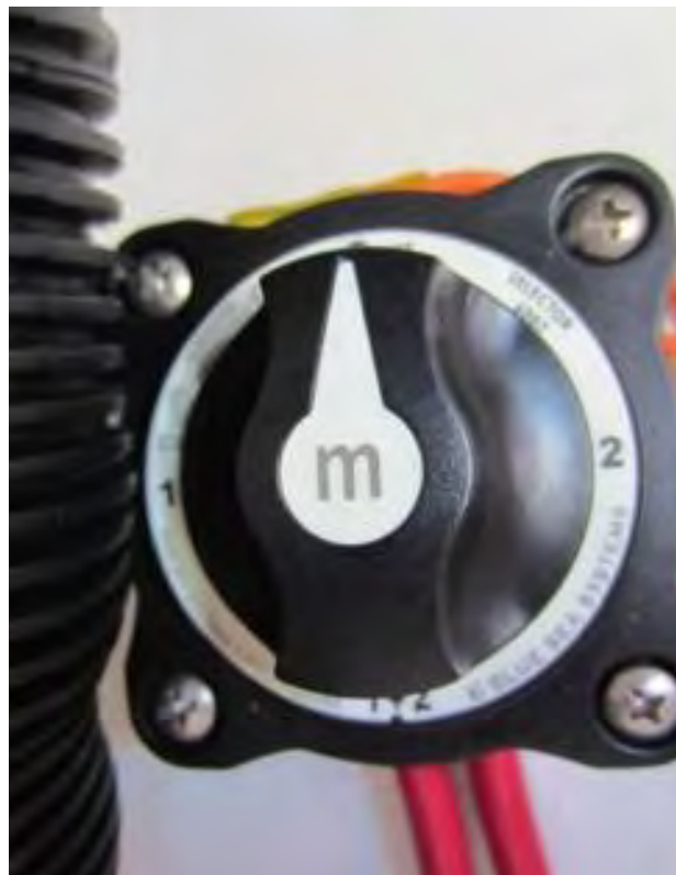
Battery Switch, Shown in the “Off” Position
