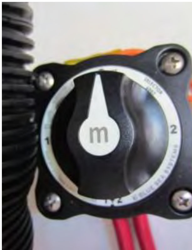
Battery Switch, Shown in the “Off” Position
