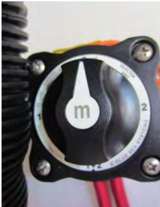
Battery Switch, Shown in the “Off” Position
